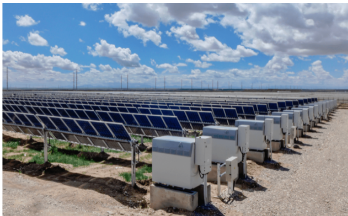
A row of vanadium flow batteries stores energy supplied by solar panels in Qinghai, China.
